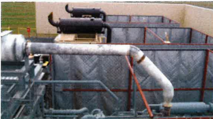
BBC-EXT-R-2" Sound Curtains enclose pumps and compressors.
